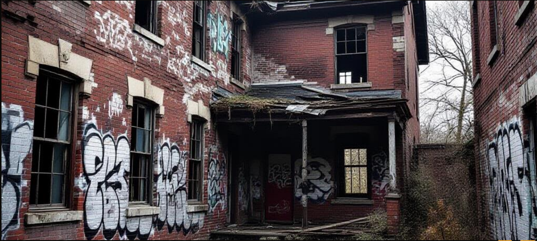
Vacant building showing signs of vandalism and structural decay, a magnet for illicit activity.
